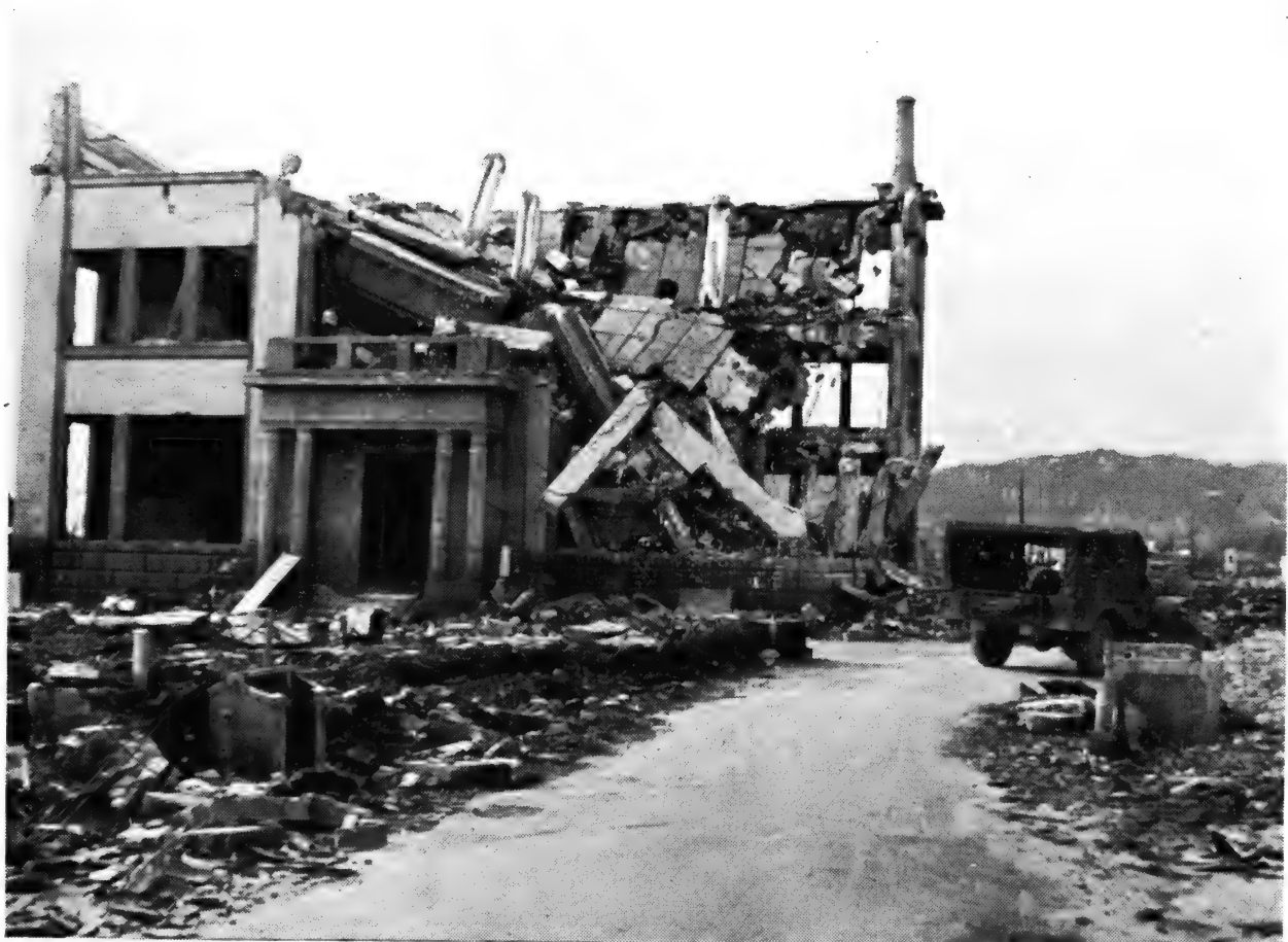
Photo No. 8. HIROSHIMA. Reinforced concrete building 200 yds. from the centre of damage, which is to the right. The blast from the bomb forced the roof slab down, the slab shearing round the column heads, leaving the internal columns projecting through the debris. Few concrete buildings failed in this way. See paragraph 24.
